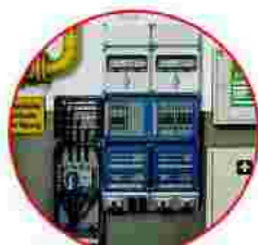
Power Distribution Panels
