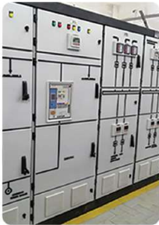
Low Voltage Switchgear
