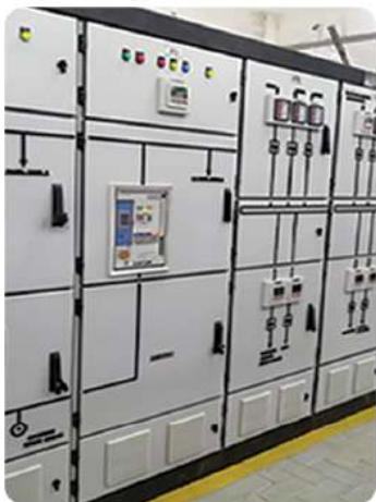
Low Voltage Switchgear
